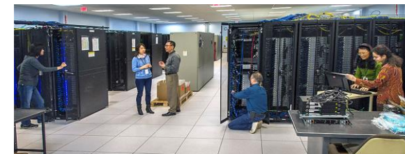
RHIC-ATLAS Computing Facility as part of the BNL Scientific Data and Computing Center.
